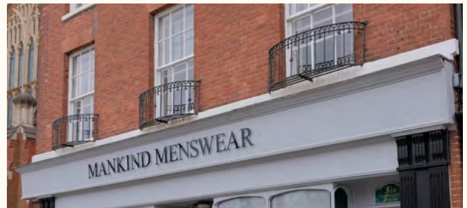
Good quality balconet design in Lichfield, which doesn't extend beyond a third of the window height, and are only marginally wider than the opening.
